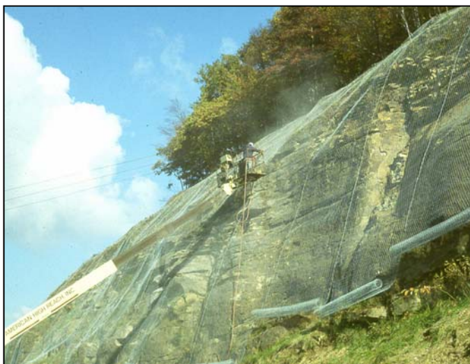
Example of Rockfall protection netting
